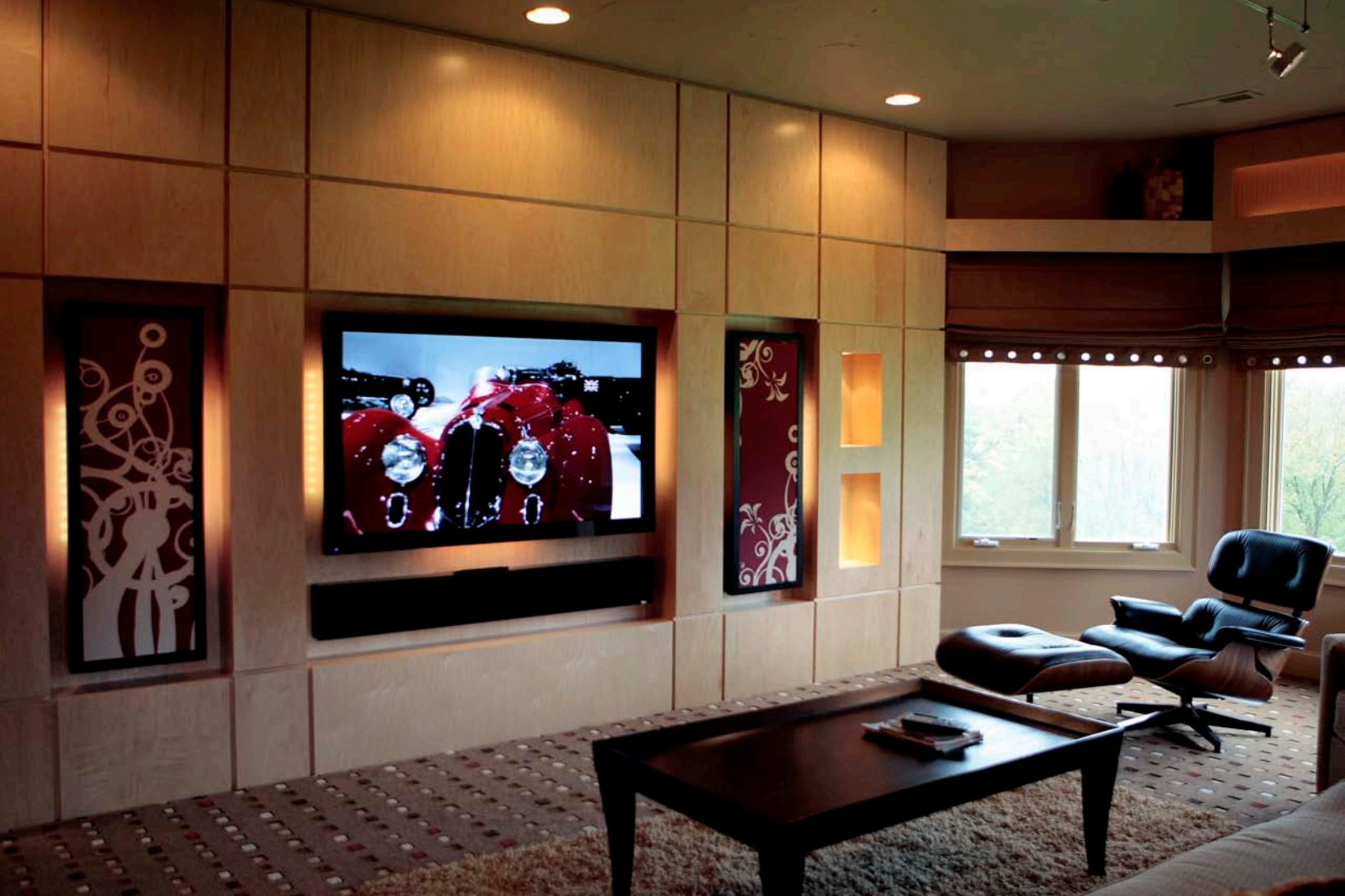
Artcoustic 5.1 Cinema Installation by Forrester Tech, Springfield, Missouri, USA
